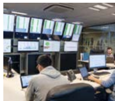
Our control room excellence is a key part in achieving EWT turbines' high availability (of 98%)
